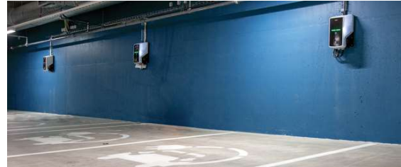
New chargers in the parking garage
