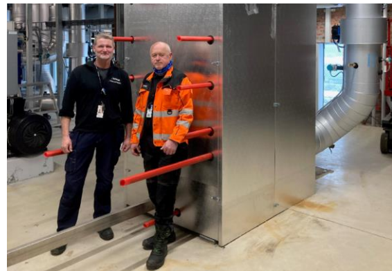
Heat exchange to wastewater in DA8.
