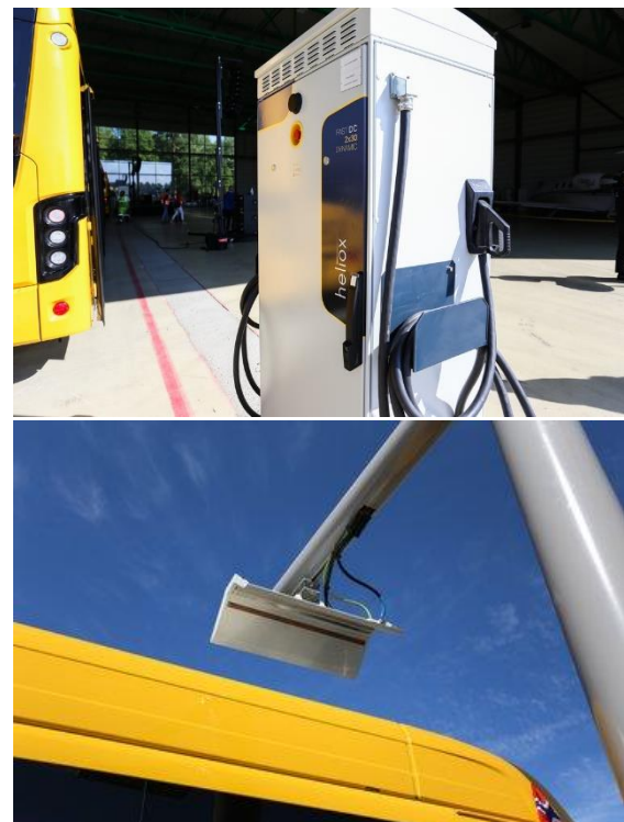
Both depot and pantograf charging.
